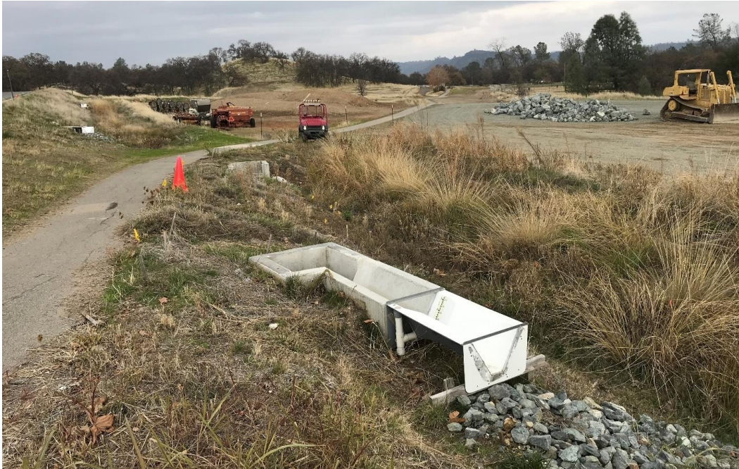
Students from Butte College and Chico State complete 12 yr project building experimental station, Biological Wetland Educational Living Laboratory (BWELL)
