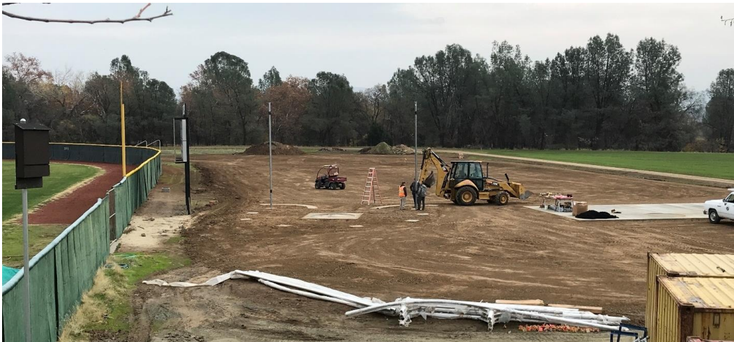
BC Sports Complex improvement project done by Tractors and Crawlers lab students
